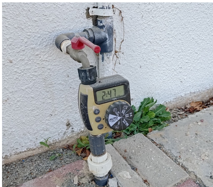
Fig 30 : Timer Switch for Irrigation landscaping at BAC-Block D
