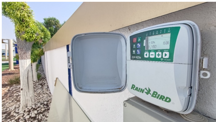
Timer Switch for Irrigation landscaping at BAC-Boundary wall
