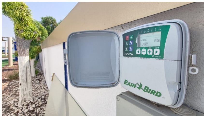
Fig 29: Timer Switch for Irrigation landscaping at BAC-Boundary wall
